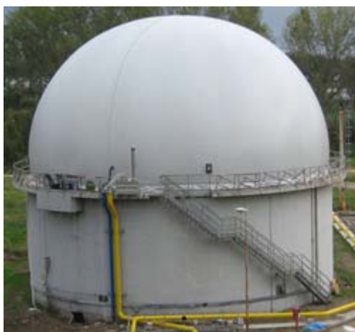
Tank roof mounted gasholder
